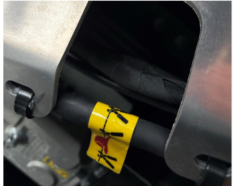
High voltage cut line
