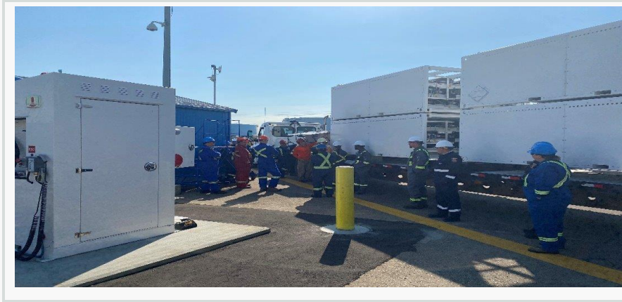
GTM, Safety Systems, Hydrogen Storage Trailer
